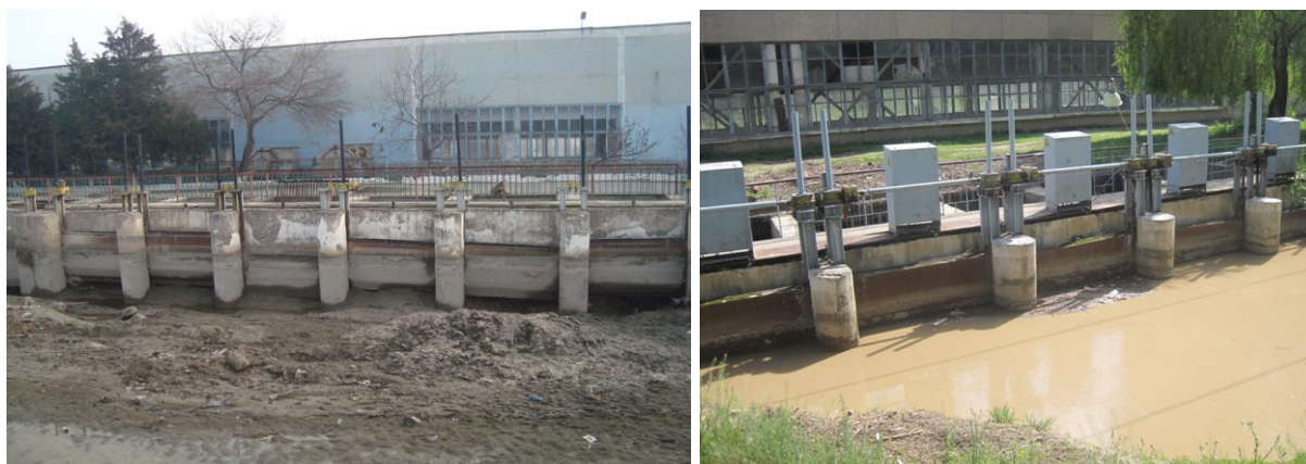
Fig. 1 - Sedimentation in the front chamber and water intake chamber of the PS “Bakht” and “Savai-1p” in the Andijan region
