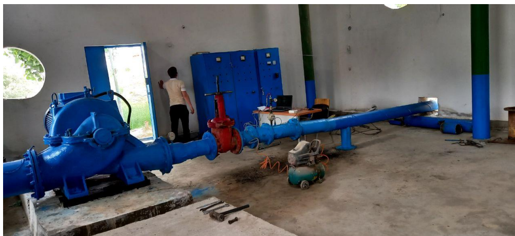
FIGURE 1. Pumping station "Kungirtag" Kashkadarya region.
